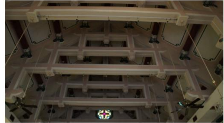
Decorative concrete beams are on the top of the church space which is imitating a Chinese wooden structure. The rose window can be seen in this photo and it is facing east from exterior.
